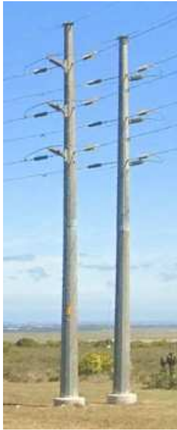
Photo 2. Typical Strain Structure (Double Pole)
