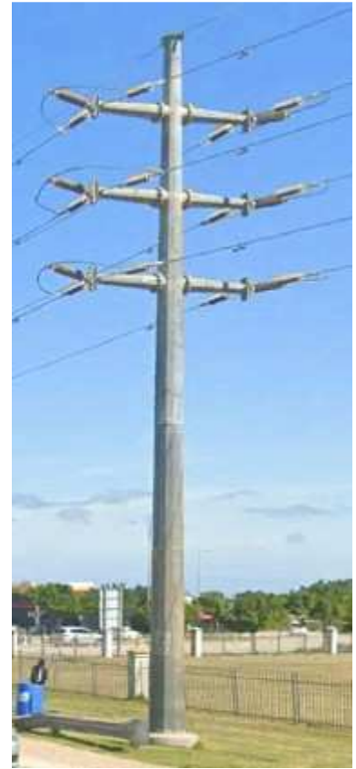
Photo 3. Typical Strain Structure (Single Pole)
