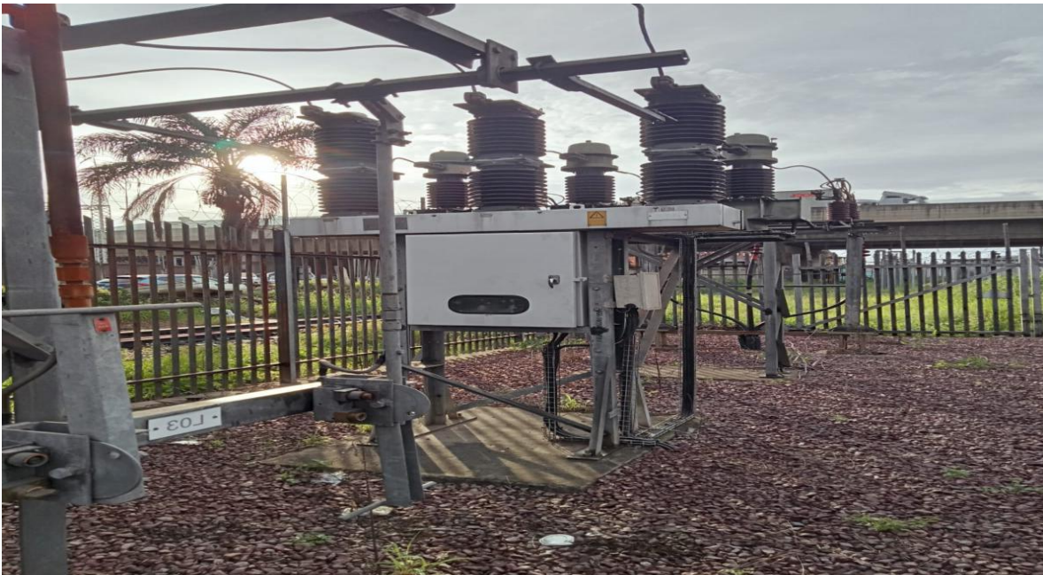
Picture 2: 33kv Primary Circuit Breaker
