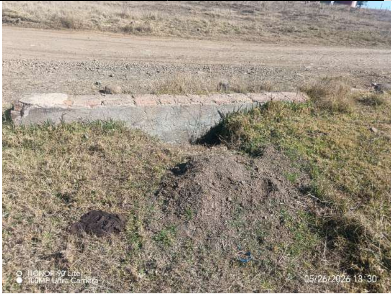
750mm circular culvert blocked
