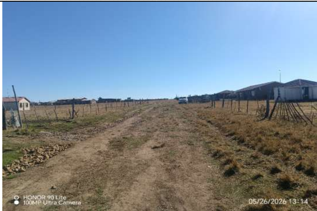
Virgin road with uncontrolled stormwater causing erosion
