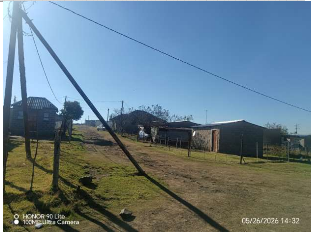
Road 1 Ward 7: Electrical stay pole to be relocated from the road way
